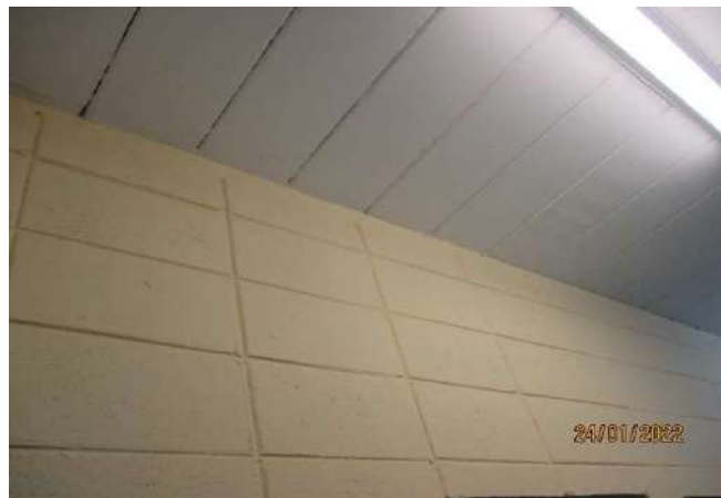
FOTO 8 PAREDE / TETO HALL PRINCIPAL
