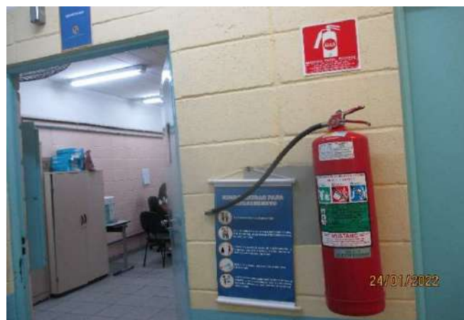
FOTO 16 EXTINTOR HALL PRINCIPAL
