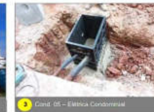
3 Cond. 05 - Elétrica Condominial
